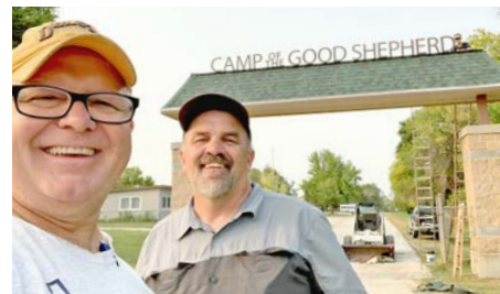
Joel, Brian and Carol (top right) complete the installation of the new CGS entryway letters.
